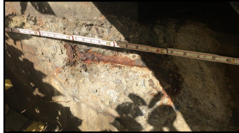
Stem Deterioration at West Abutment
