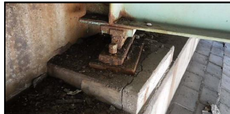
Cracked Bearing Seat
