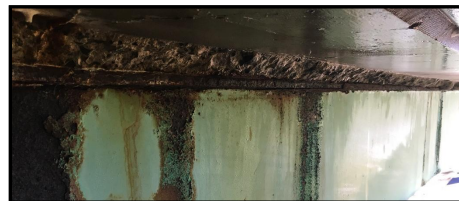
Haunch and Top Flange Deterioration
