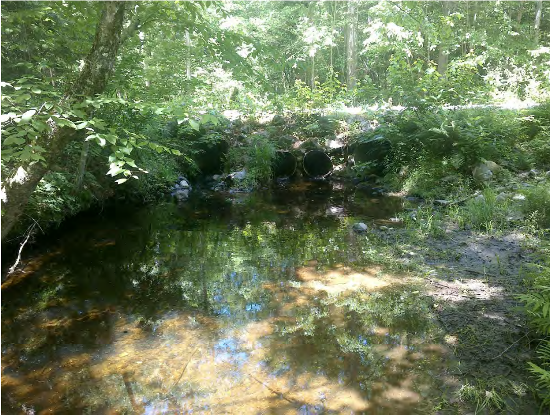
Site 4. Looking upstream at four culverts and over-widened somewhat unstable channel.
