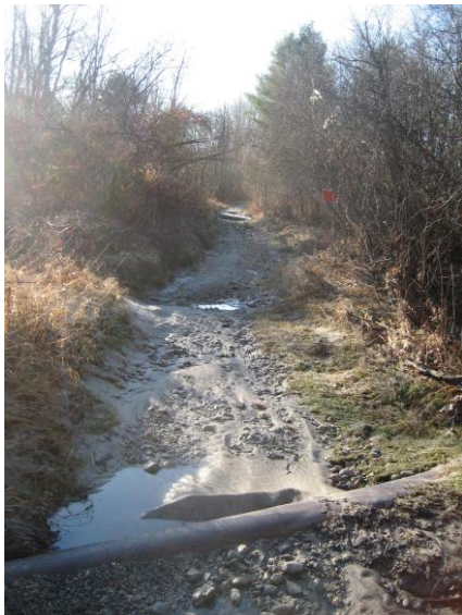
The CMP access road along the river is heavily washed out. It needs to be relocated.
