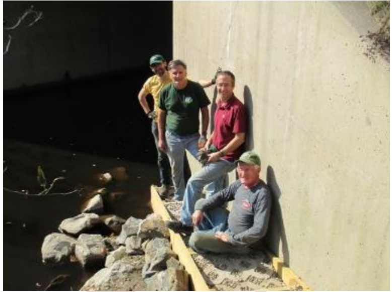
Photo 10 Volunteers work on a canoe launch to improve access to the East Branch Conservation Area.
