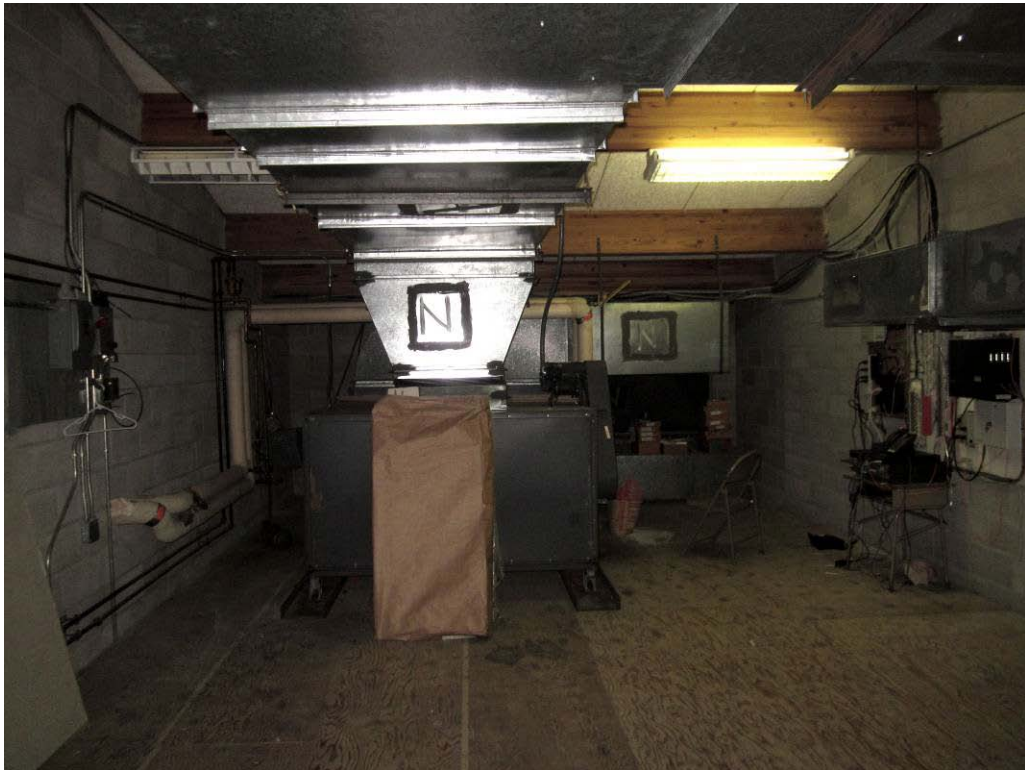
Photo 22 – Existing ventilation unit
