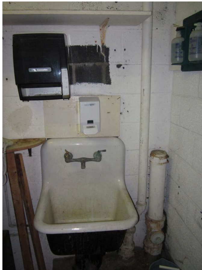
Photo 20 – Existing janitor's sink in electrical room
