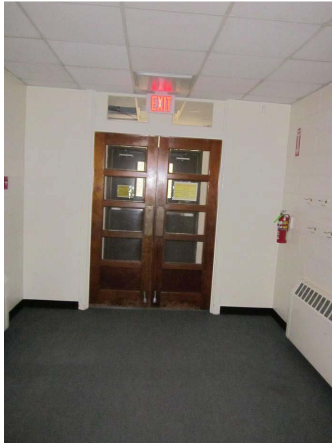
Photo 8 – Existing egress doors – non-ADA compliant size
