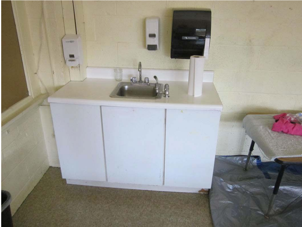
Photo 11 – Existing classroom sink and cabinet – non-ADA compliant
