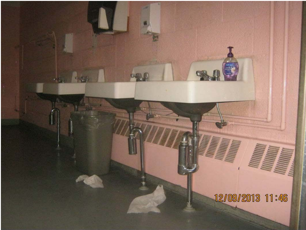
Photo 14 – Existing women’s room – non-ADA compliant fixtures and accessories
