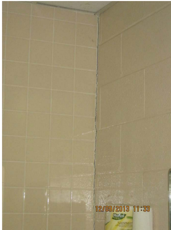
Photo 15 – Existing locker toilet room – movement crack
