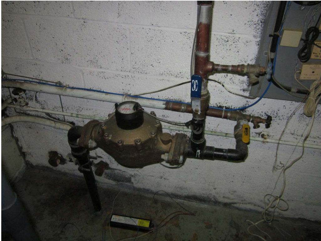
Photo 21 – Existing domestic water entrance
