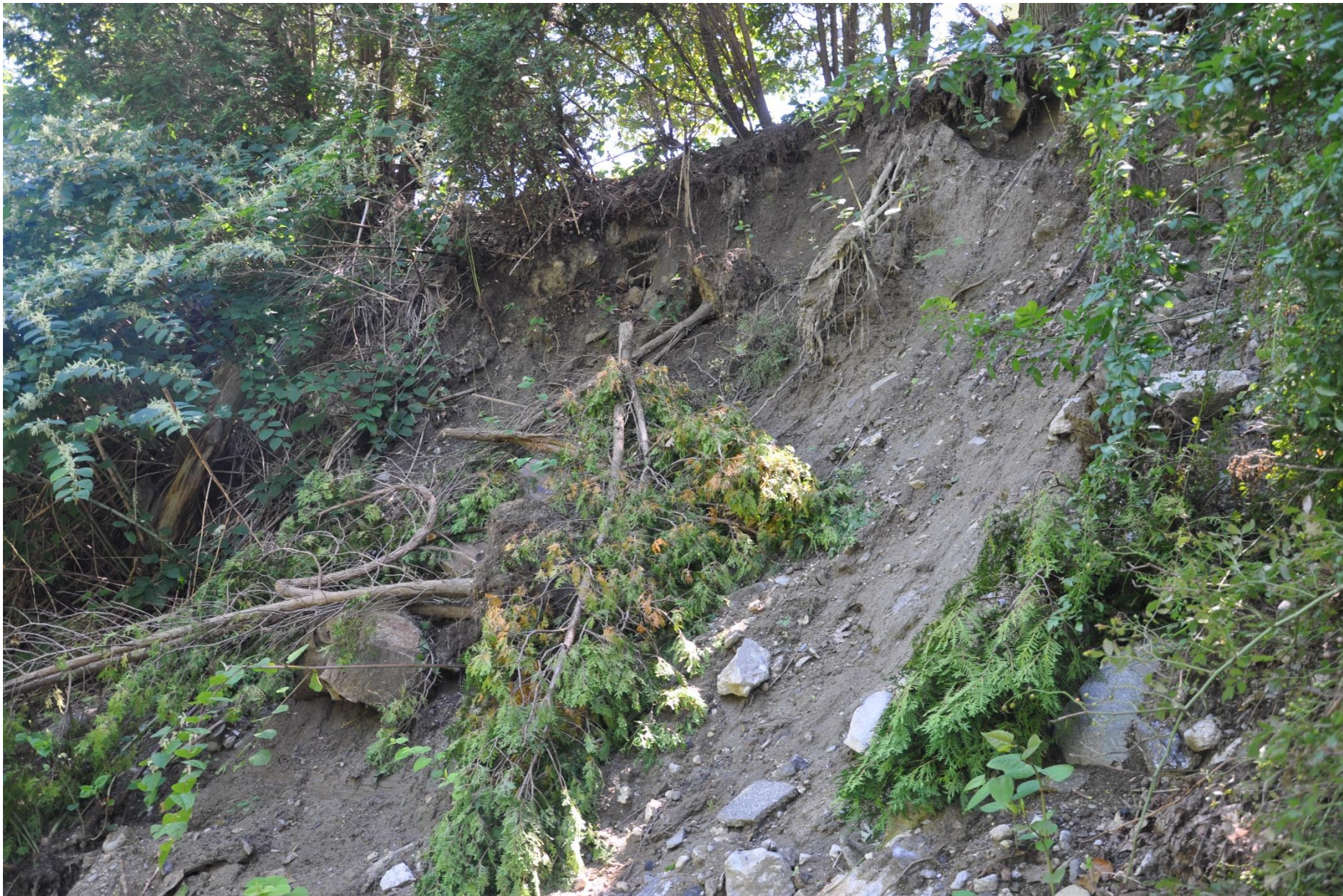
SITE PHOTOGRAPH – COLLAPSED SLOPE
