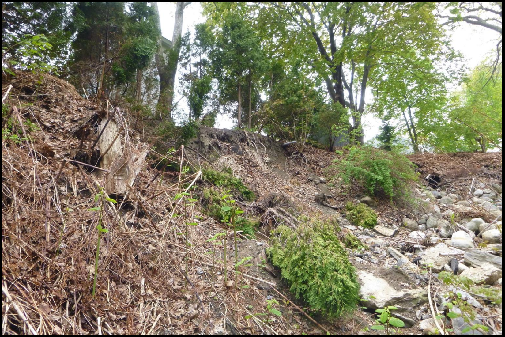
5.2015 Slope erosion below outfall
