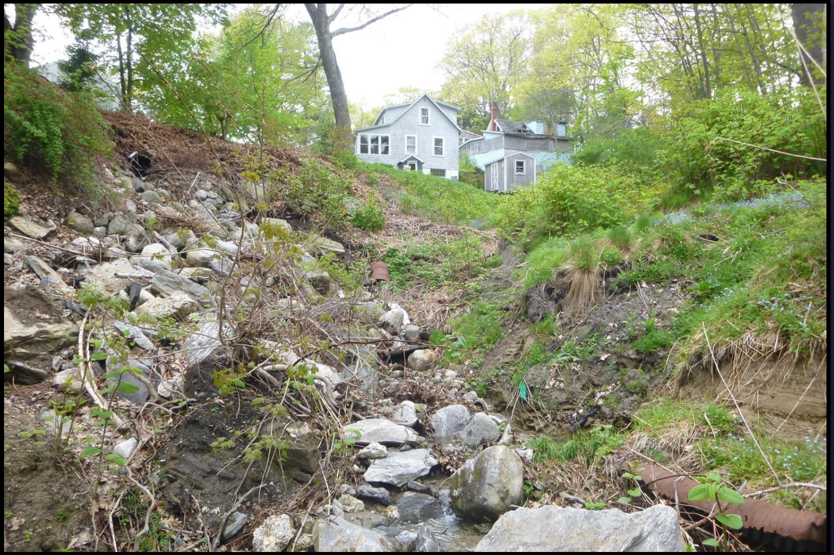
5.2015 Erosion below outfall
