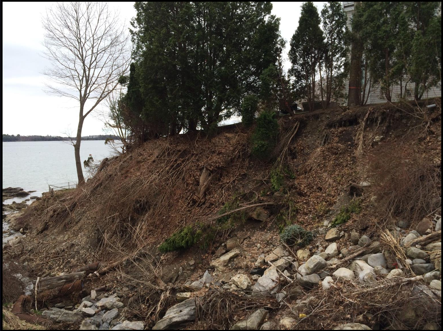
5.2015 Slope Erosion adjacent to Cohen Propety
