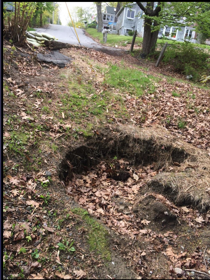
5.2015 Sinkhole on Stormwater Discharge Route
