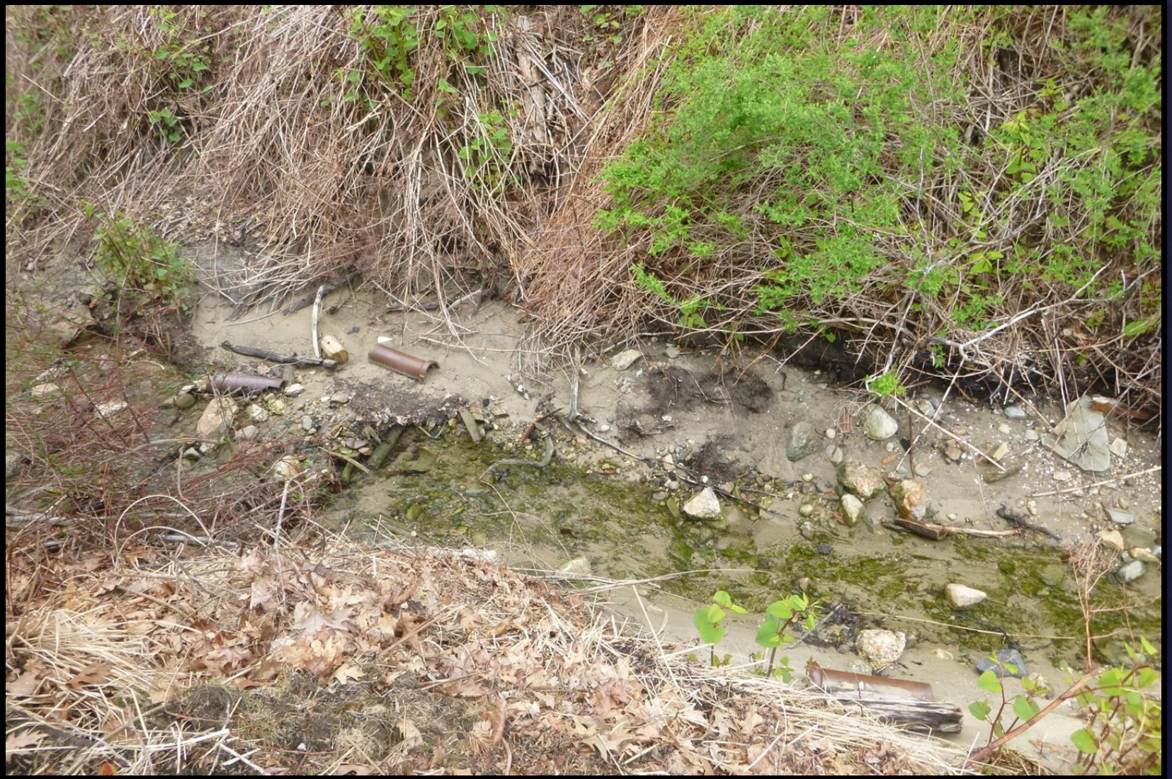
5.2015 Drainage Channel washout below outfall
