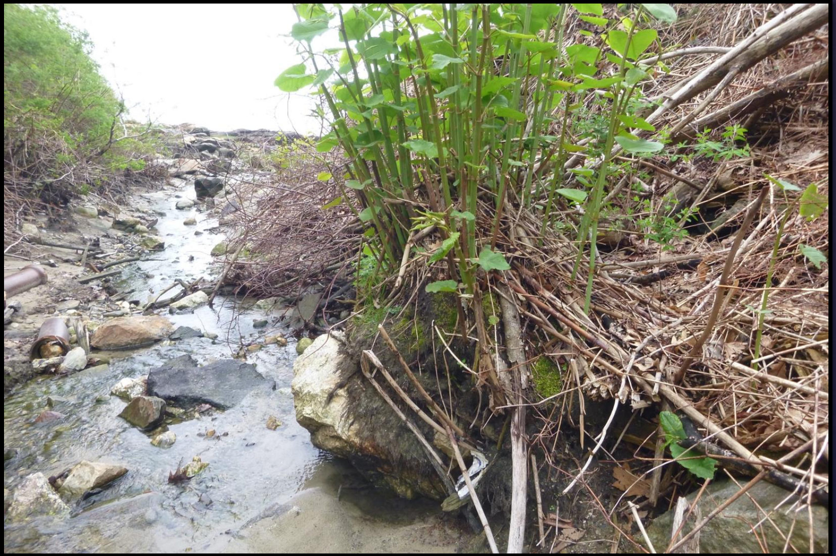
5. 2015 Drainage Channel washout below outfall (2)
