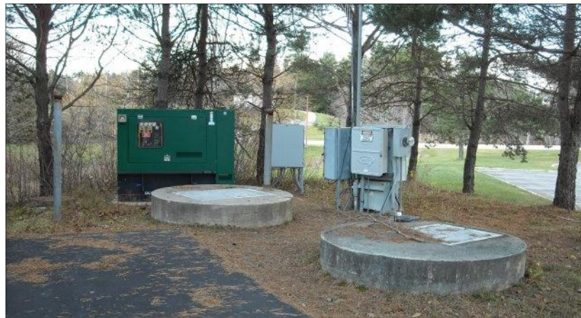
FIGURE 2-5 WOODLAND CLUBHOUSE PUMP STATION
