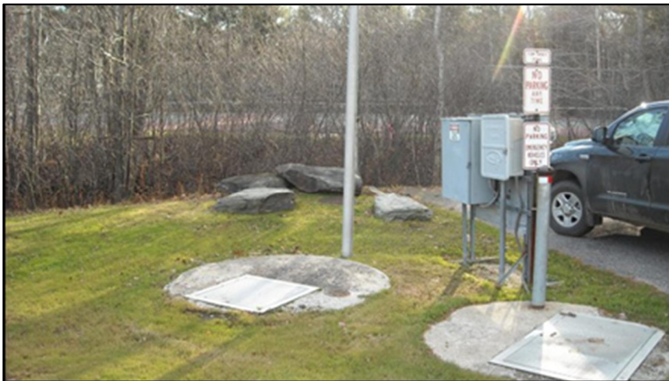
FIGURE 2-8 HIGH SCHOOL PUMP STATION
