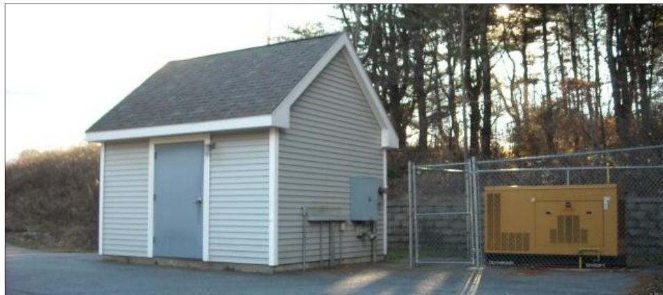
FIGURE 2-9 FALMOUTH ROAD PUMP STATION
