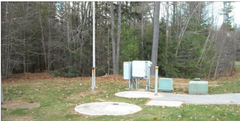
FIGURE 2-7 WOODLANDS DRIVE PUMP STATION
