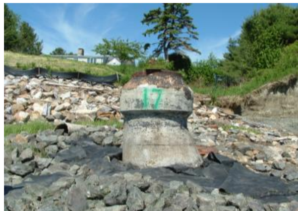
Raised manhole along Shoreline Drive in need of additional reinforcement against tidal action
