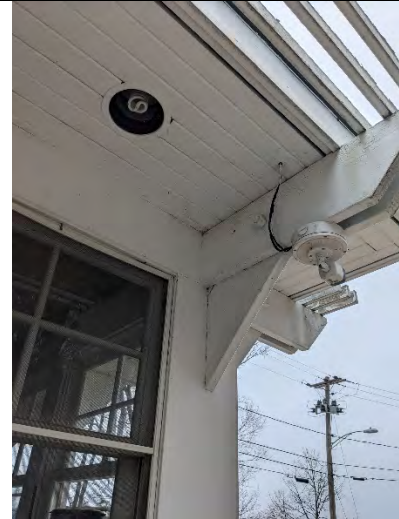
Ext Lighting and Security Camera
