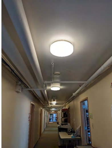
Existing Light Fixtures
