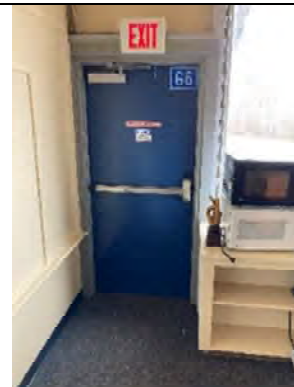
Non-ADA compliant approach at exterior door.
