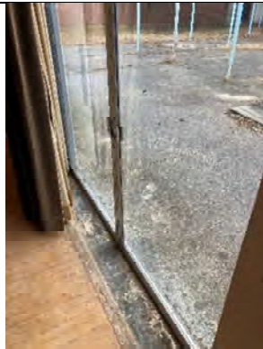
Moisture penetration at exterior doors.
