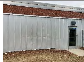
Damaged metal siding.
