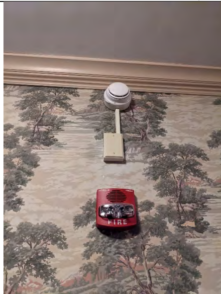
Fire Alarm Devices
