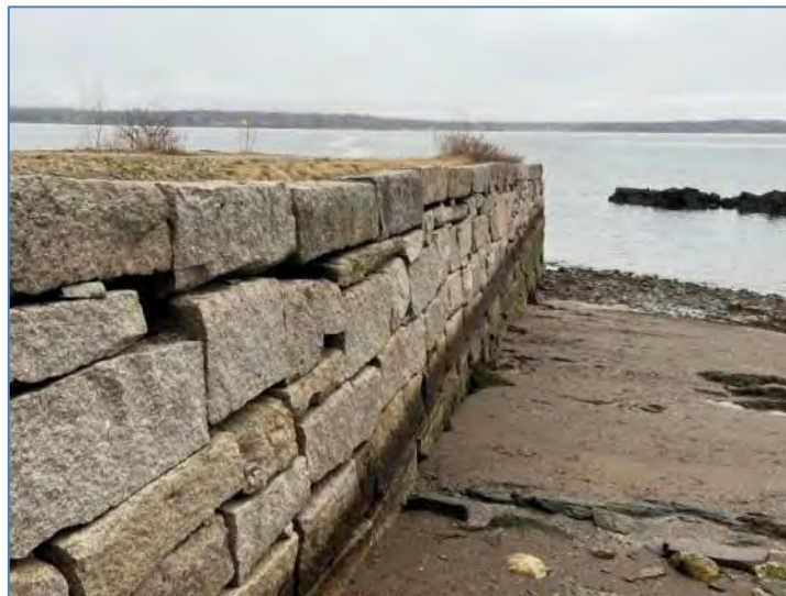
Fig. 12. Granite Pier at Low Tide (Remnants offshore suggest the original pier extended into deep-water)
