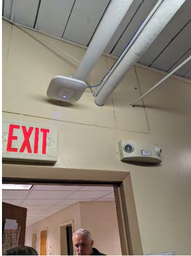
Exit Sign, WAP, Battery Light
