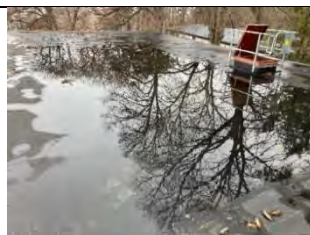
EPDM Roof ponding
