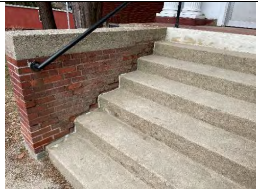
Mortar deterioration near door A2
