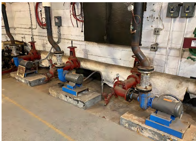
Figure 7 - Main Heating Pumps
