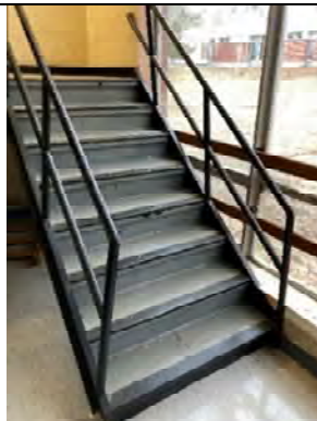
Egress Stair with non-compliant railing system.
