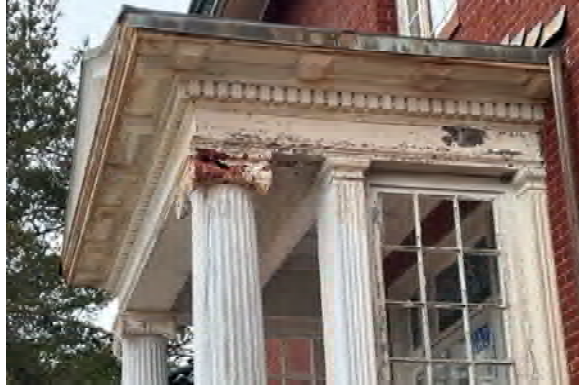
Wood deterioration near door A2
