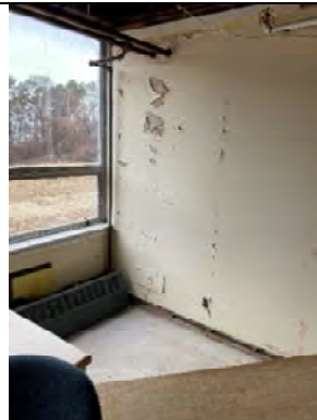
Deterioration at existing partition wall.
