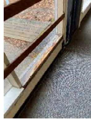
Water damage at sill.
