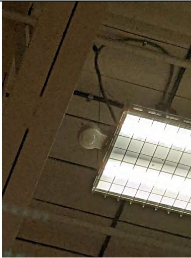
Gymnasium fixture with Controls
