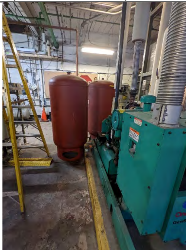
Generator Adjacent to Expansion Tanks
