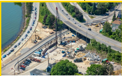
Week-long full closure of Veranda Street. No travel to Portland via Route 1. Detour to Middle Road.
