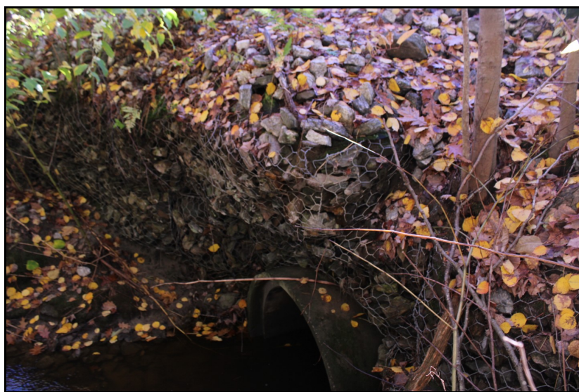
Figure 33. Gabion baskets on the headwall of Northbrook Drive are sliding down slope above the culvert inlet.
