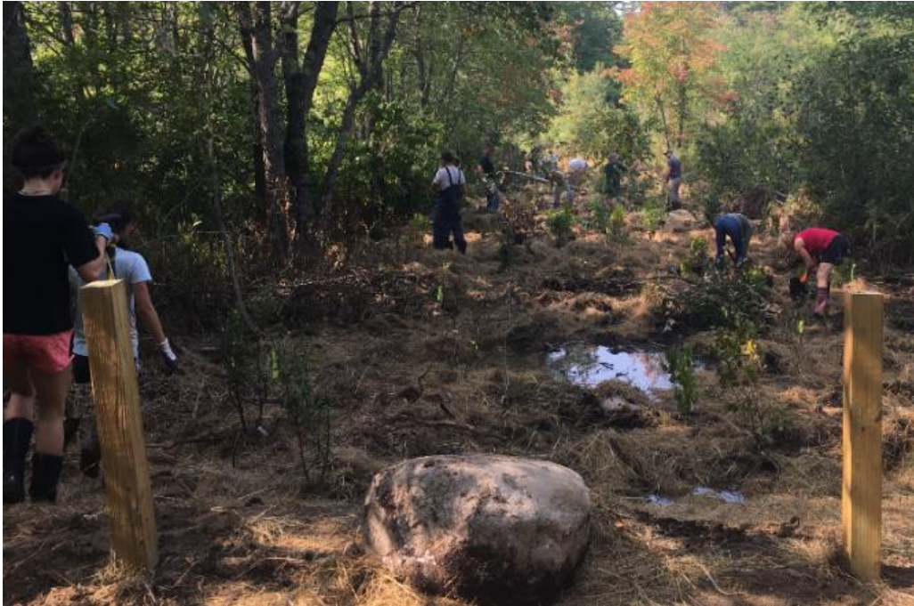
Photo 5 Members of the Falmouth Conservation Corps install plantings in restored wetland adjacent to Highland Lake on the McDermott Way parcel in the Suckfish Brook preservation area.
