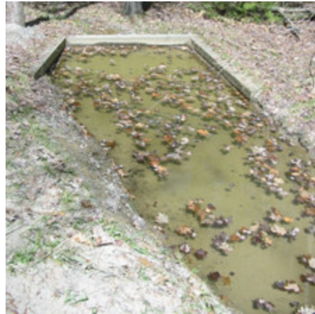
The above photo shows a typical level spreader used to evenly disperse flows to a vegetated area.
